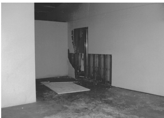
Figure 9.16 Vapor explosion blast damage.
