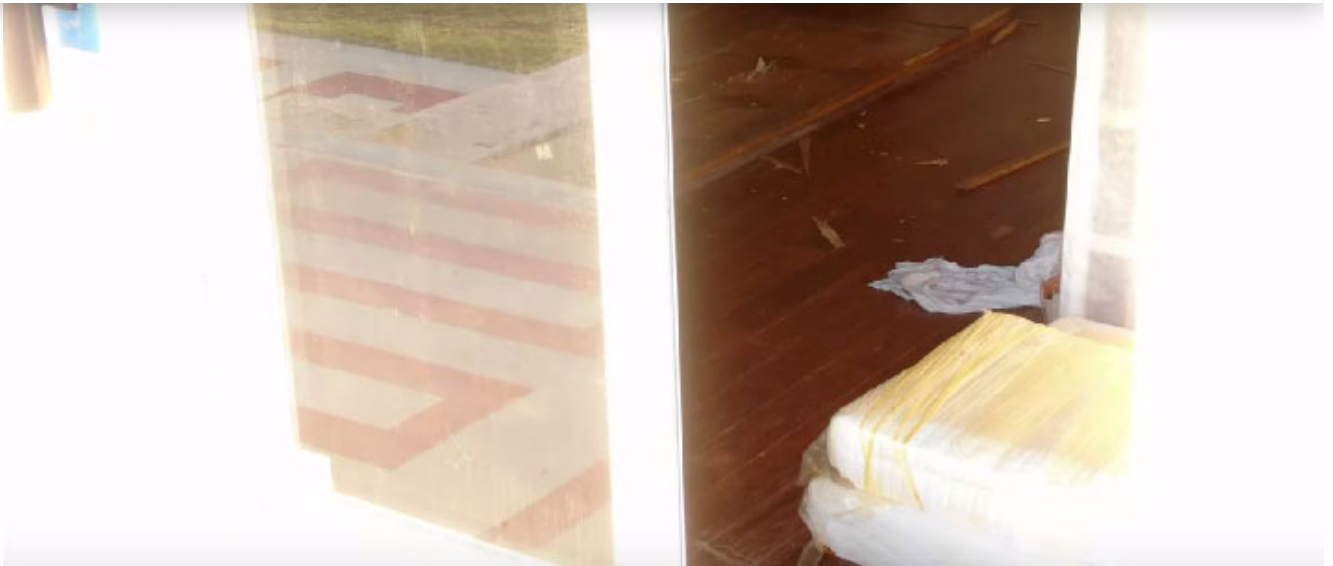
Here, we see wooden floors and broken wood pieces. .
