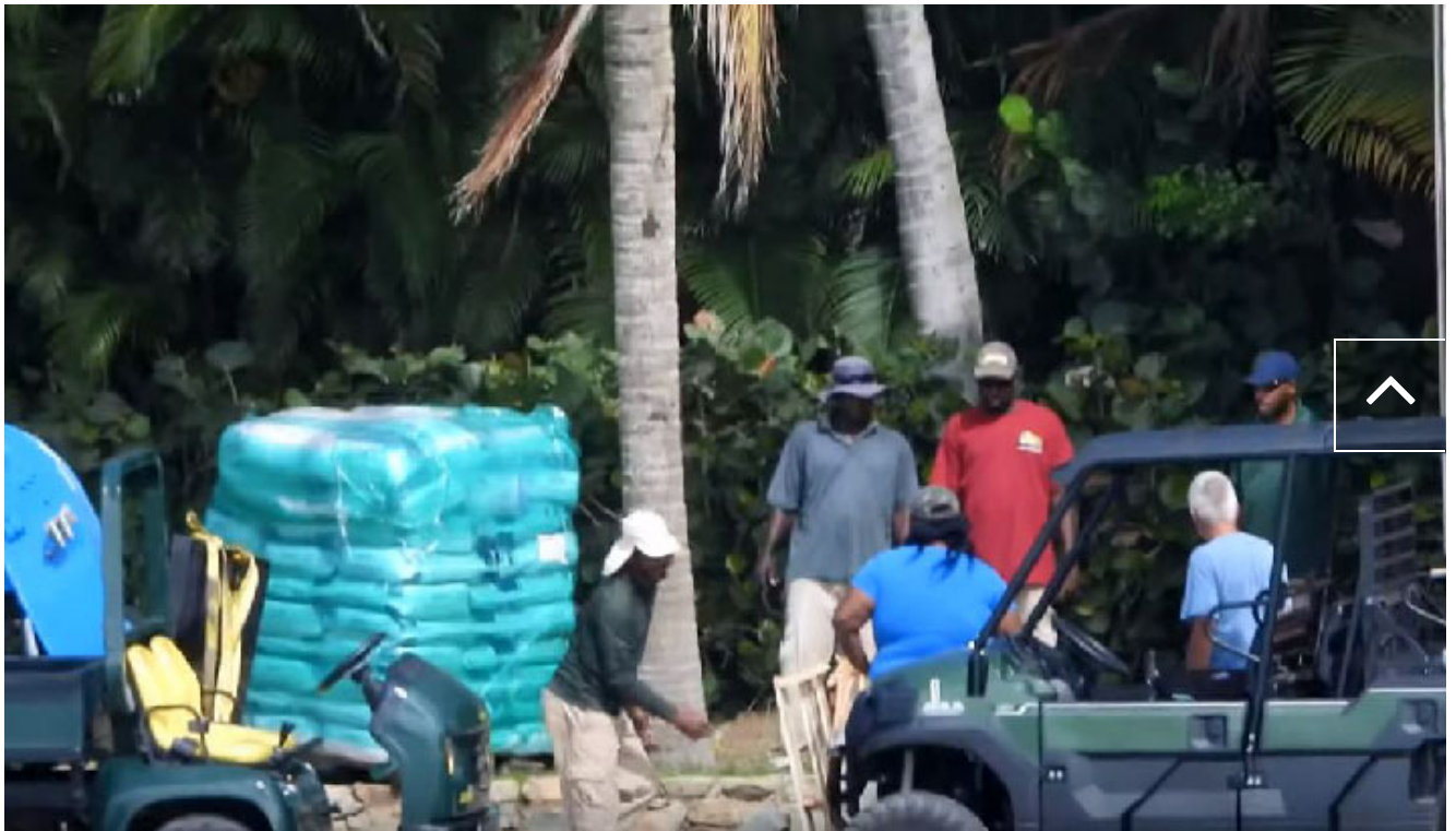
This footage was filmed on July 30th, 10 days before Epstein's death and 12 days before the FBI can see construction workers, heavy machinery and bags of material, possibly concrete.
